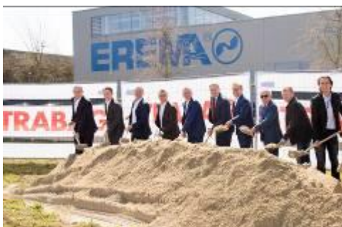
Photo 3: Ground-breaking for the construction of additional production and office space at the company headquarters in Ansfelden.
